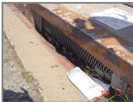
Figure 3.7 Typical opening cover after Rain Event No. 3 (2/17-18/06)
