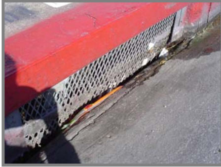
Figure 3.8 Typical opening cover after Rain Event No. 4 (3/19-20/06)
