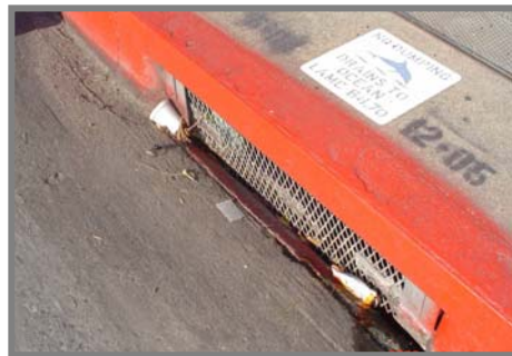
Figure 3.6 Typical opening cover after Rain Event No. 2 (12/31/05 – 01/02/06)
