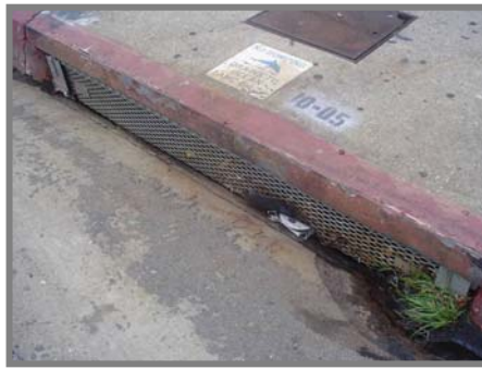
Figure 3.5 Typical opening cover after Rain Event No. 1 (10/17-18/05)
