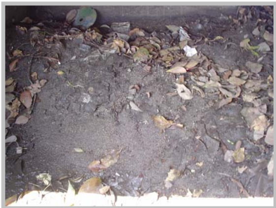
Figure 3.3 Typical CB insert with sediment in catchment area
