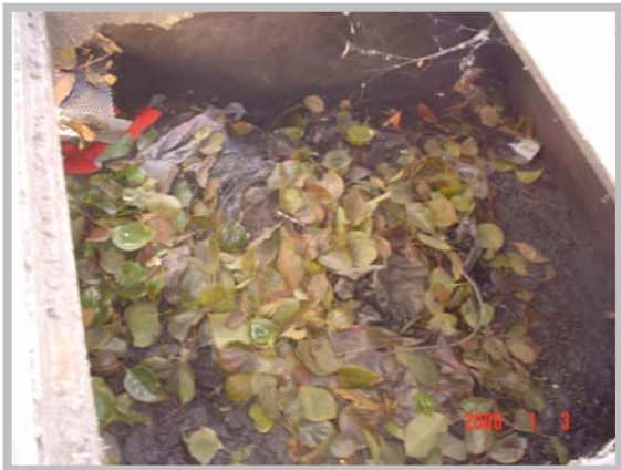
Figure 3.2 Typical CB insert with vegetation in catchment area
